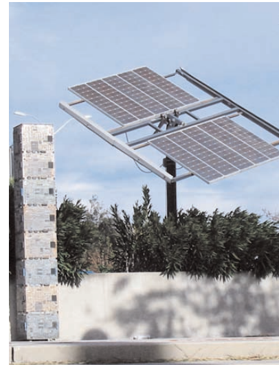
Photovoltaic installation at north campus entrance
